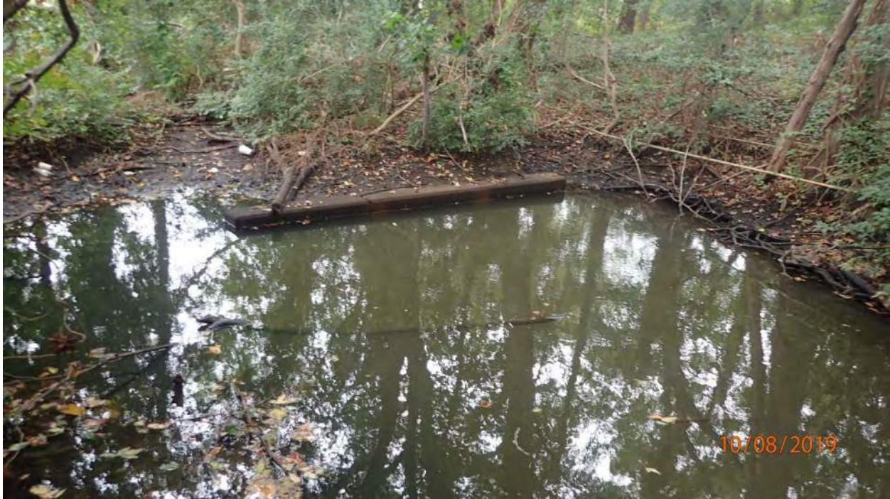
Photo 3 – Waterway WL002 in Area 19, facing north (upstream) at culvert that extends under 1 st View Street
